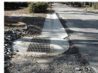
The new gravity storm-drain system discharging to the pump station consists of double drop inlets and piping along Broad Bay Road.
