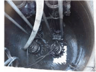
Float controls activate the pumps based on the water level inside the manhole. Two pumps operate simultaneously during heavy flooding.
