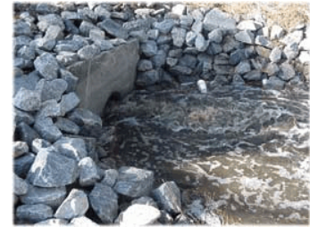
Riprap placed at the gravity outfall pipe helped control erosion from the increased discharge.
