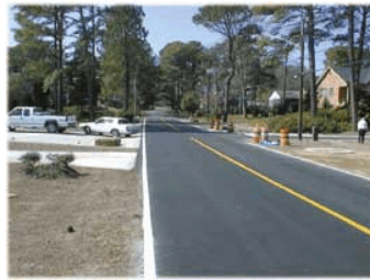
During the drainage improvement project, the City of Virginia Beach worked with residents to provide road and landscape improvements in the area.
